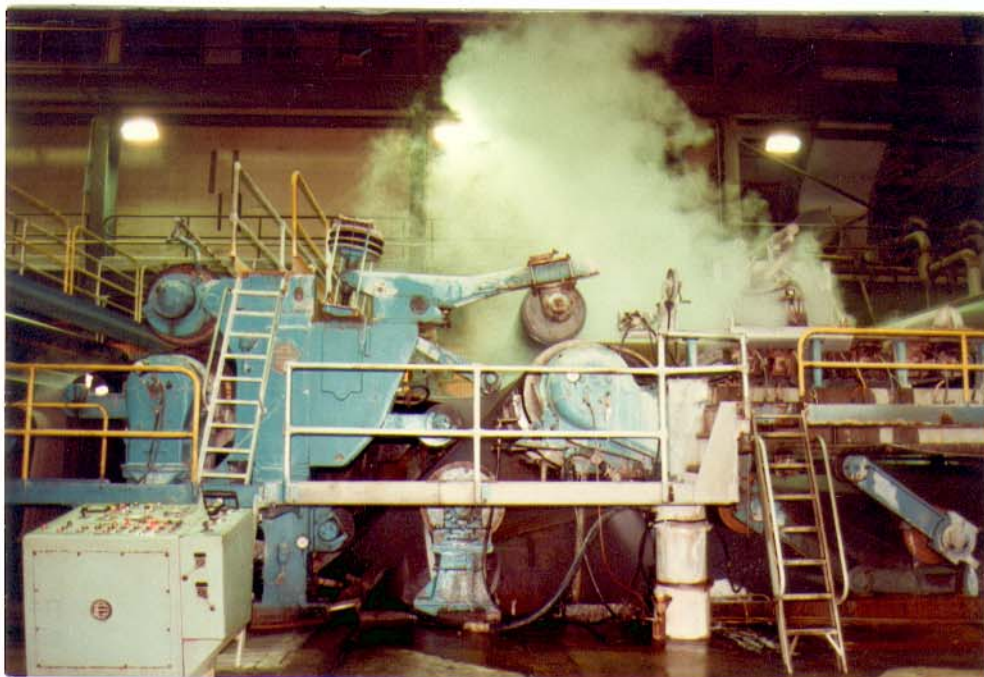
Picture of Water Vapor & Corrosion Before Installation
